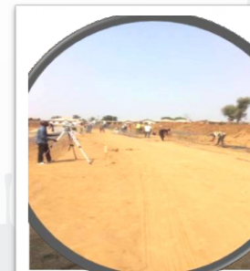
Ongoing development of site and Serviced Plots at Apata Yakubu, Ilorin, Kwara State.
