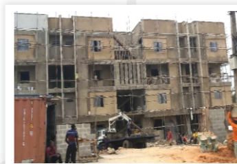
Ongoing Construction of 8 Units 4 Bedroom Maisonette at 36, Bankole Crescent, Adeniyi Jones, Ikeja
